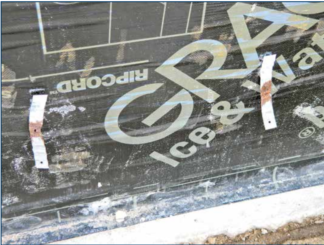
Figure 5 – These inexpensive veneer connectors within an unventilated cavity wall on a spec office project that was never occupied are only six years old. Notice the premature corrosion on the veneer connectors.
