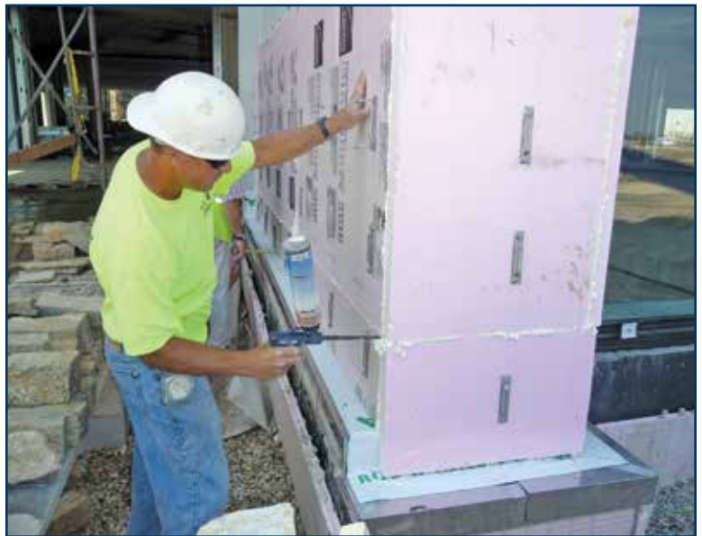
Figure 8 – Wall insulation joints being foamed to make thermal control layer continuous and prevent air from circulating between insulation and support wall.
