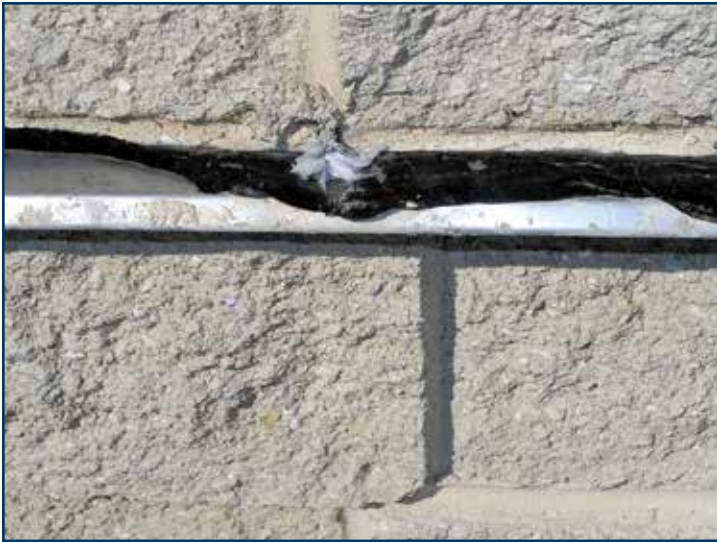
Figure 10 – Rope wicks like this polyester rope with cotton surround do not allow air into the wall cavity and are not very effective at letting water out of the wall cavity because about 80% of the rope does not have wicking properties. Furthermore, cotton rope wicks have been known to petrify when cement-laden moisture works through them.
